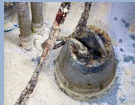
One of two SE pumps for pumping wastewater containing chemicals with large variations in pH from the CIP process at a dairy producing cheese.
